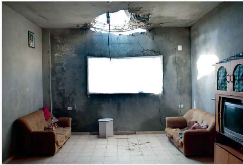
Traces of roof-penetrating munitions. Tuffah, Northern Gaza, 2009. Being able to study similar strikes in Gaza assisted the analysis undertaken remotely in Pakistan. KENT KLICH
